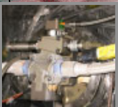
Pressure Transducers and Fill Valves
